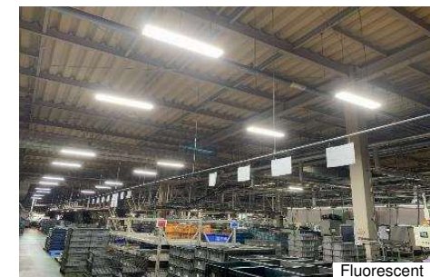
Completed installation of LED lighting in production areas Plans to expand to office area in the future
